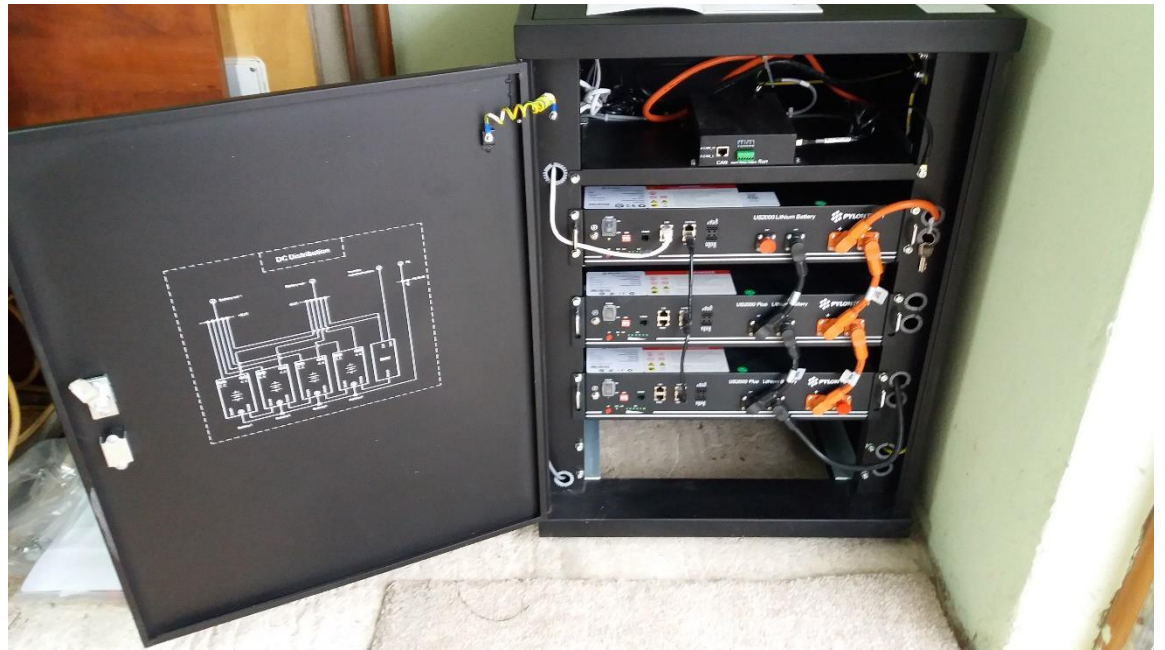
Picture shows 3 x 2.4kWh lithium batteries in a cabinet, making the storage capacity of 7.2kWh. Accessible to increase the capacity in blocks of 2.4kWh. This battery system can be adapted to work with grid connection and off the grid applications because of its 48v circuit.
